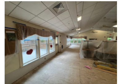
The Norfolk Facilities Department has managed contract restoration services. Some repairs include tearing down and re-doing the insulation and walls of the Senior Center following a pipe burst that caused significant damage to the building in February.
