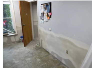
The walls at the Senior Center have since been fixed and are ready to be painted.
