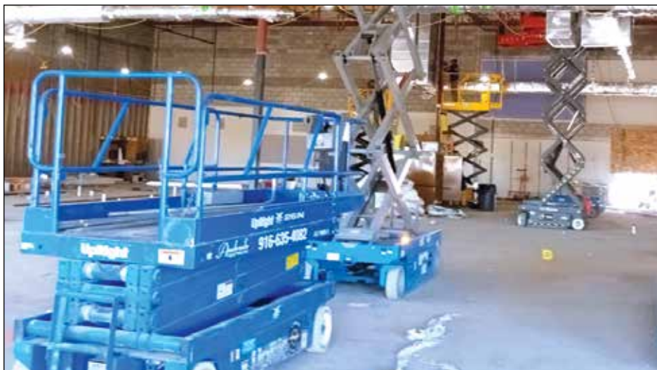
Interior work being conducted on the new plasma center at the former Dimples Records store at 7830 Macy Plaza Drive in Citrus Heights.
