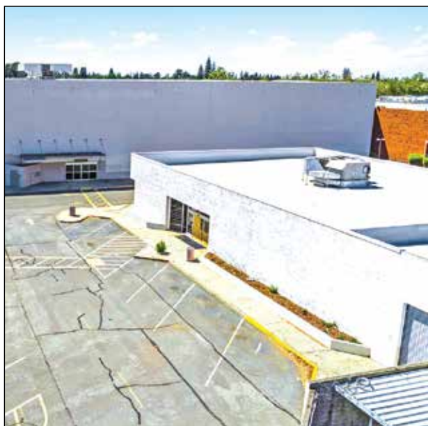
Colliers Retail Capital Markets image of Sunrise Mall Sears building now listed for sale for $8 million. Photo courtesy of Sunrise MarketPlace
