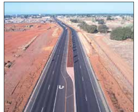
The White Rock Road Phase Two project is a 1.5-mile, four-lane segment of White Rock Road from Fitzgerald Road to approximately one half-mile east of Rancho Cordova Parkway in order to alleviate traffic congestion. Photo courtesy of City of Rancho Cordova
