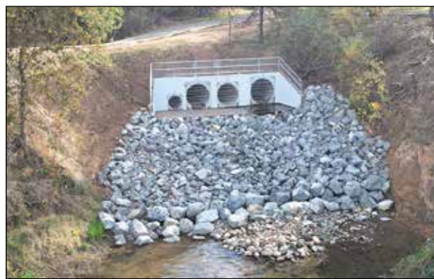
In the American River Outfall Four Repair Project the City rehabilitated a 45-year-old damaged storm drain outfall near Ambassador Park. Photo courtesy of City of Rancho Cordova
