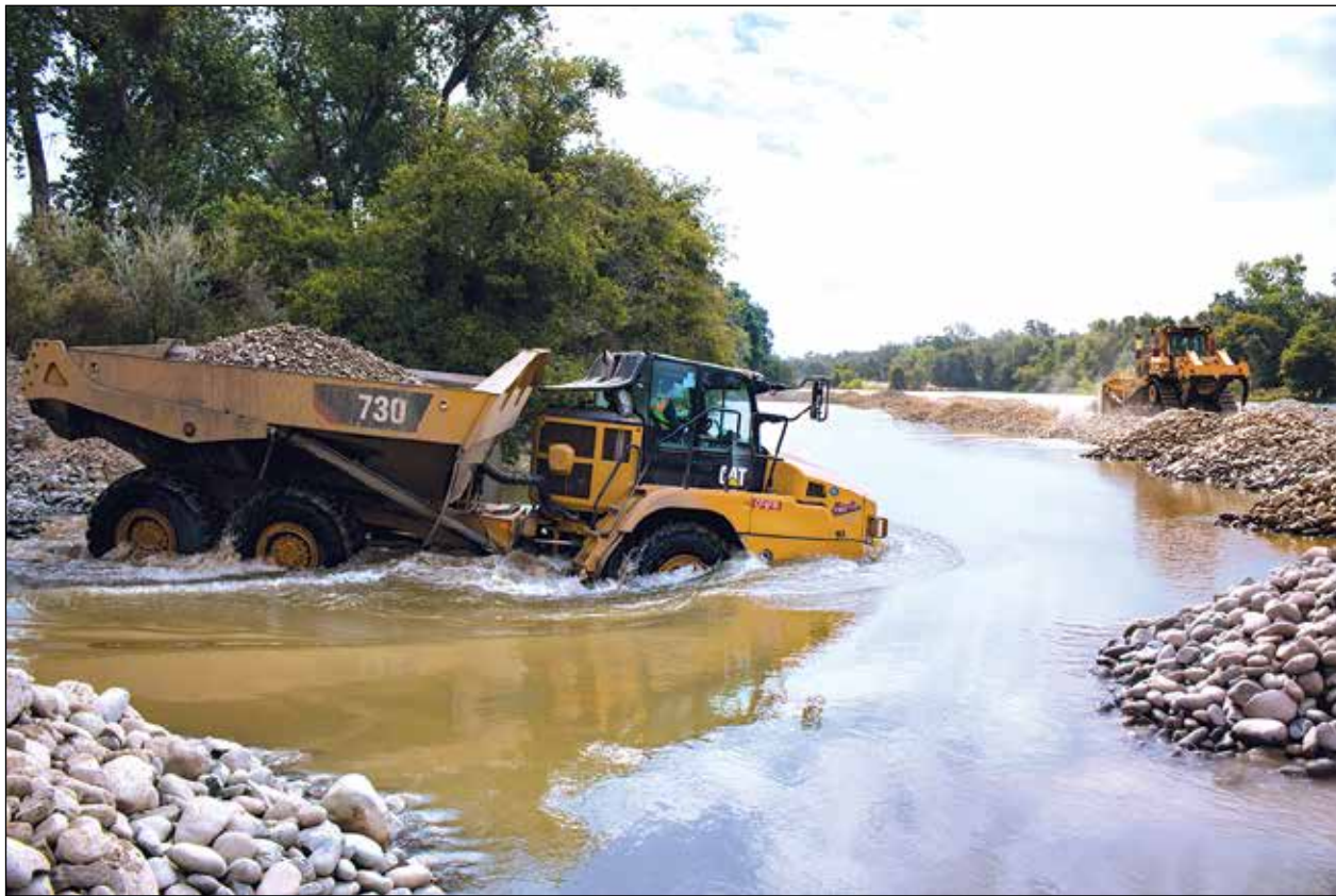
Sacramento City utility crews move gravel into Fair Oaks reaches of the American River. Two Sailor Bar locations – and a third site below Nimbus Dam – are being restored to enhance salmon and steelhead spawning.
