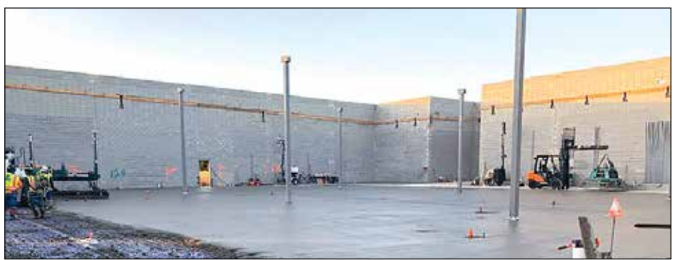
The 23,000-square-foot cinder block structure for the future Sprouts at Stone Creek Village is rapidly being finished. Photo courtesy of City of Rancho Cordova
