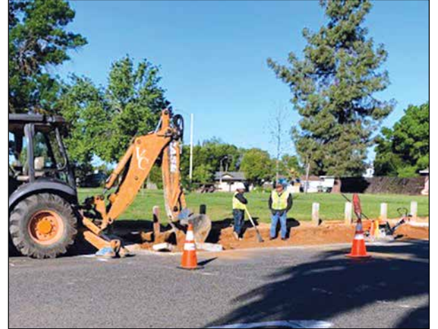
Cordova School Zones projects are envisioned to support various modes of transportation. Photo courtesy of the City of Rancho Cordova
