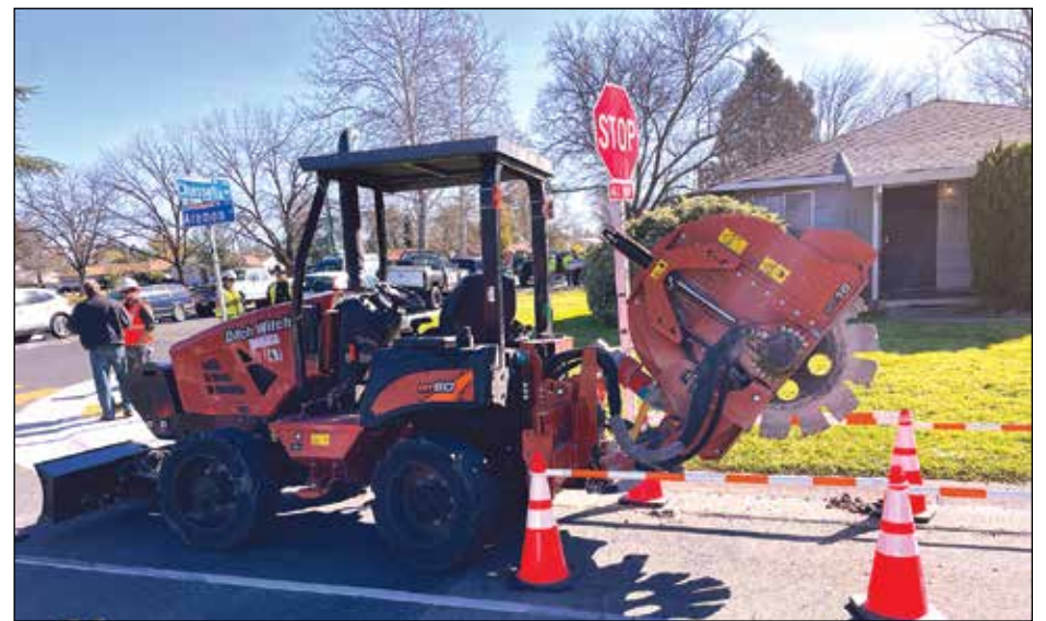
The micro-trenching machine will be used to make trenches for the fiber cables around the city. Photo by Doug Benton
