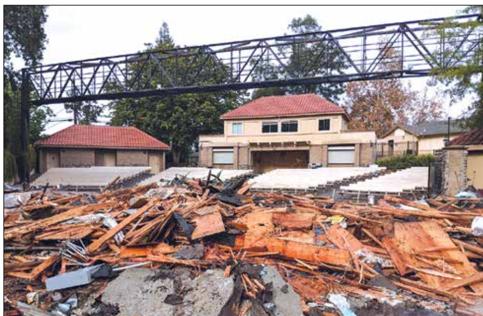
On October 7, the Fair Oaks theatre building was demolished, making room for the planned renovation, which is funded by the Measure J bond.
