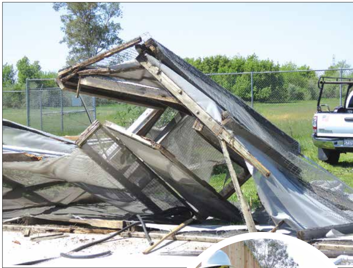
Above: February's gusty winds did some serious damage. Right: Volunteer workers employed by Wells Construction Corporation erect new walls for the Sacramento Wildlife Care Association's new aviary. Photos by Cecilia Lee Feser
