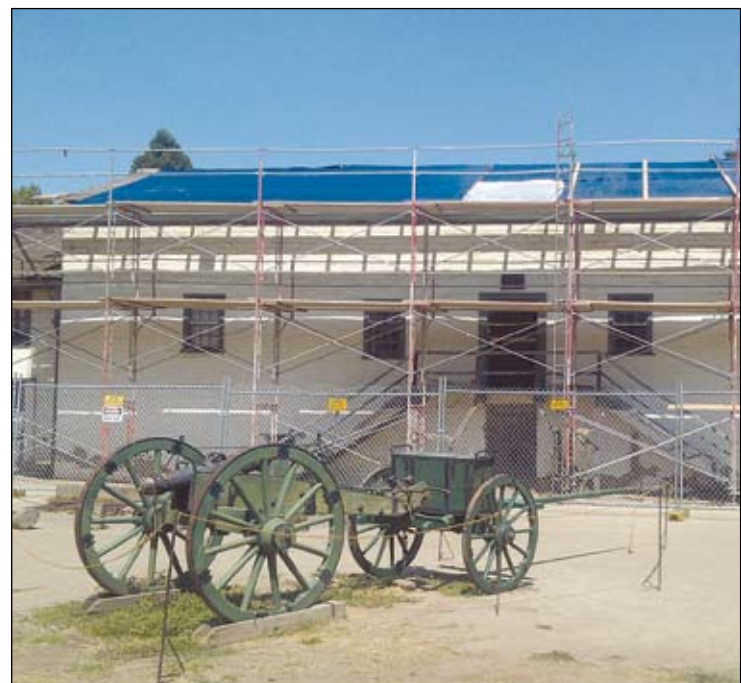
First Phase of Project Includes New Roof & Wall Stabilization for Historic Structure Originally Built in 1840.
