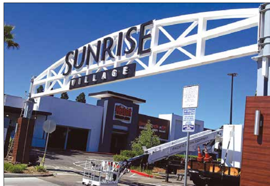
A new gateway arch to the plaza from Sunrise Boulevard greets shoppers to the newly remodeled and expanded Sunrise Village Shopping Center.
