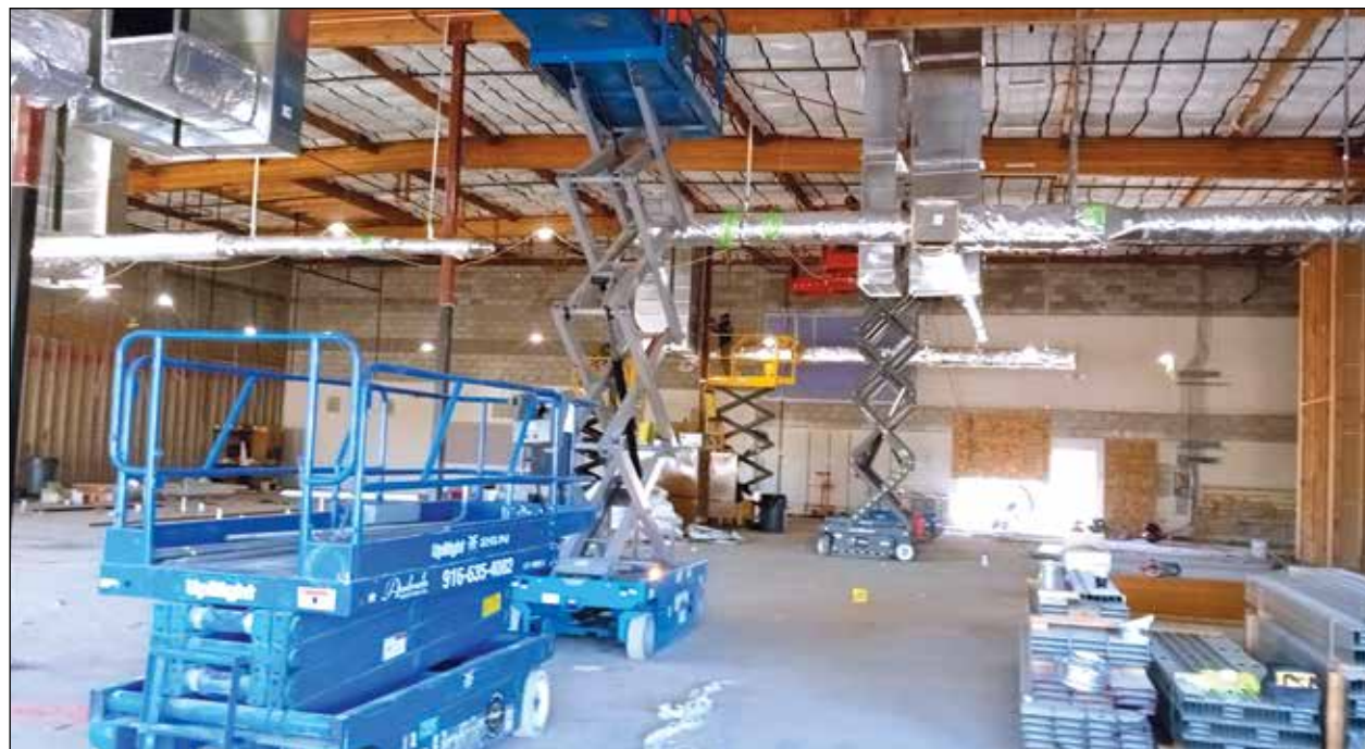
Interior work being conducted on the new plasma center at the former Dimples Records store at 7830 Macy Plaza Drive in Citrus Heights.
