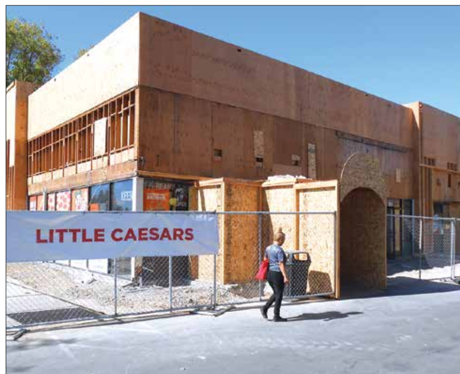
Several retail shops and restaurants, such as Little Caesar's pizza, will remain open as construction continues.
