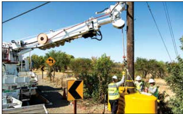
SMUD has seen an increase in "car-pole" accidents in recent years, so the electric utility is installing some measures to mitigate damage to power poles and other electrical equipment. The work is part of SMUD's efforts to enhance public and worker safety and the SMUD grid's reliability. Photo courtesy SMUD
