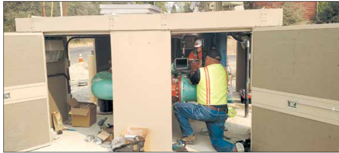
PCWA Water Distribution Operator Don Miller conducts testing alongside the construction crews. Photo courtesy of Placer County Water Agency
