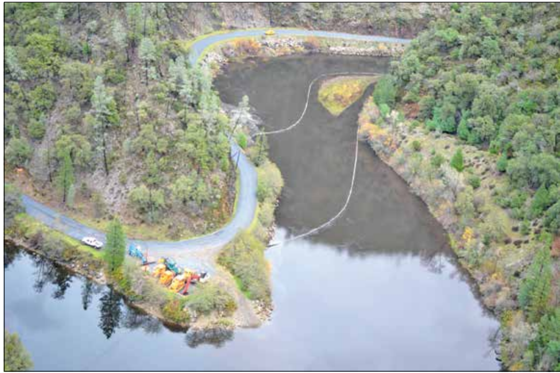
Log booms have been anchored and placed to keep logs and debris from the King Fire from washing into Placer County Water Agency's (PCWA) Ralston Afterbay.
