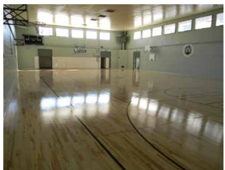
Photo of Gym After Facelift.. Photo Credit: Sheryl Petersen, Recreation Services Manager, Auburn Recreation District
