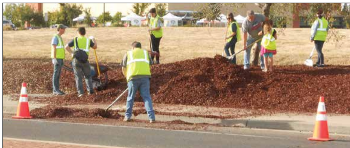
Volunteers spread approximately 2,200 yards bark along 3,000 linear feet of landscaped beds along the side of Fountain Square Drive.
