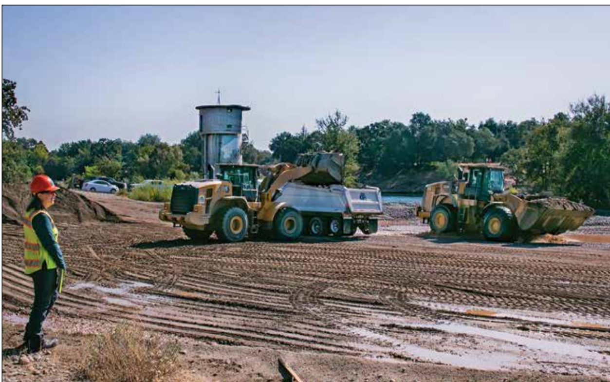
Carmichael's iconic water tower stands amid the $3.6 million project to restore salmon spawning beds on the American River. Water Forum Habitat manager Erica Bishop watches excavation progress near Ancil Hoffman Park.
