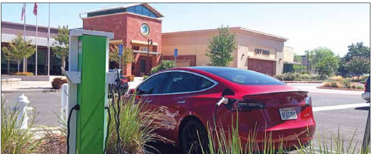
Citrus Heights City Hall has two stations (4 ports) for charging electric vehicles and is working on possible additions of stations on site.
