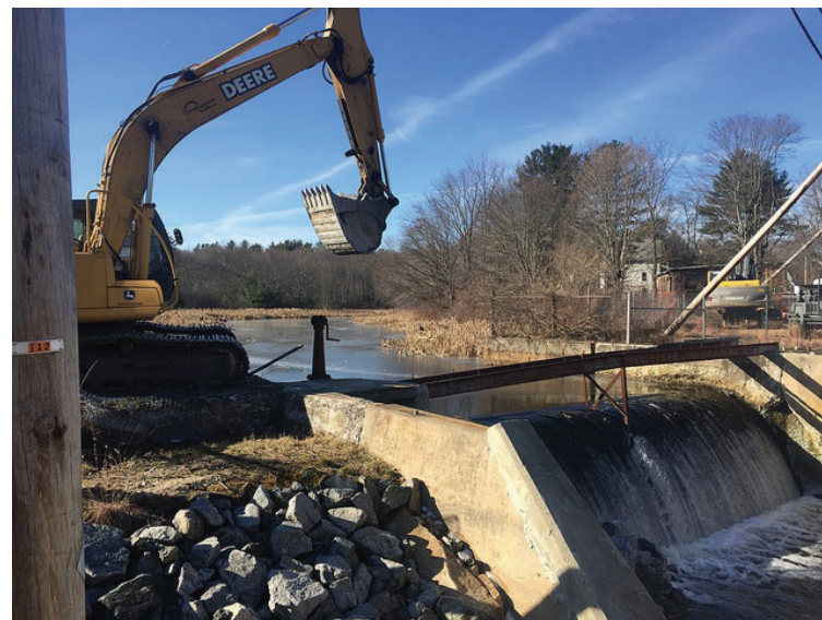
The North Bellingham Dam, a relic of industrial mill days, interrupts the natural ecosystem. Hopes are that its removal will restore natural order as well as create wetlands that protect from flooding.
