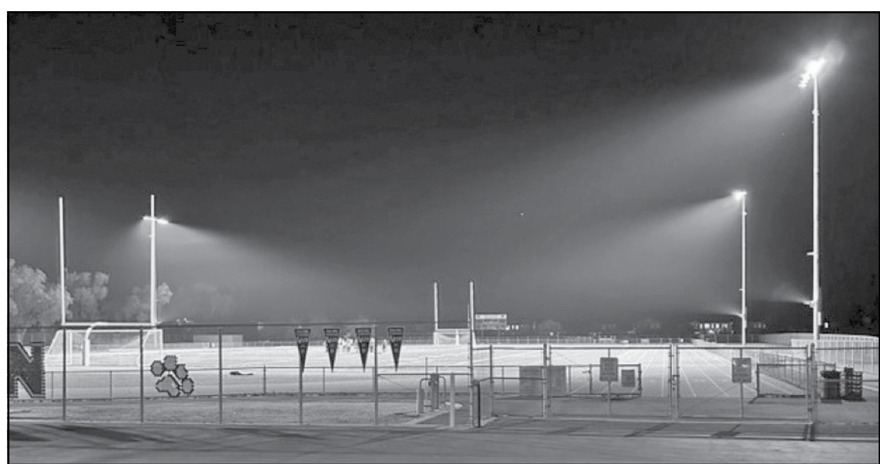
The lights are now on at Franklin High School's on-campus athletic facility. All nine of the comprehensive high schools in the Elk Grove Unified School District now have lights installed at their football/soccer/track facilities. Courtesy Franklin High School
