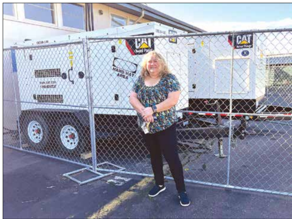
Anderson Elementary School Principal Rayito Farris stands in front of two generators providing electricity to the school. There is a third near the school cafeteria. "We have to look for the silver lining," she said. "There has been so many challenges for adults and children."
