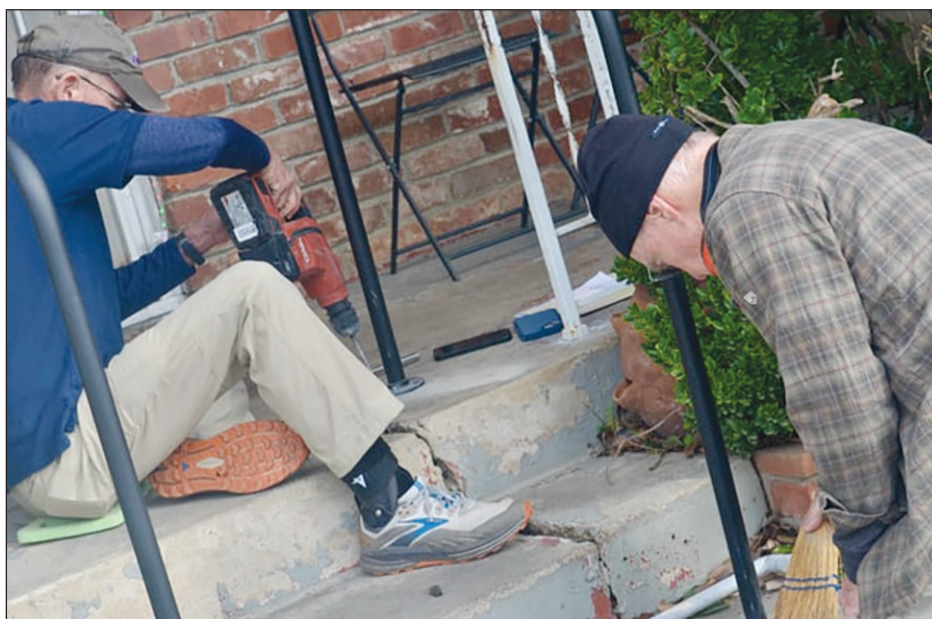
Safe at Home volunteers Dan Ward, of Carmichael, and Stan Jones, of the Greenhaven/Pocket area, install a handrail for a Sacramento resident in need of safer step way. Photo courtesy of SAFE Credit Union
