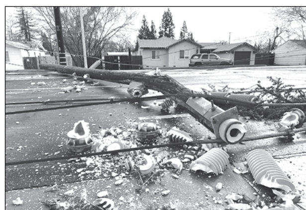
SMUD crews were out in full force to repair damage caused by the high winds. Photo courtesy SMUD.
