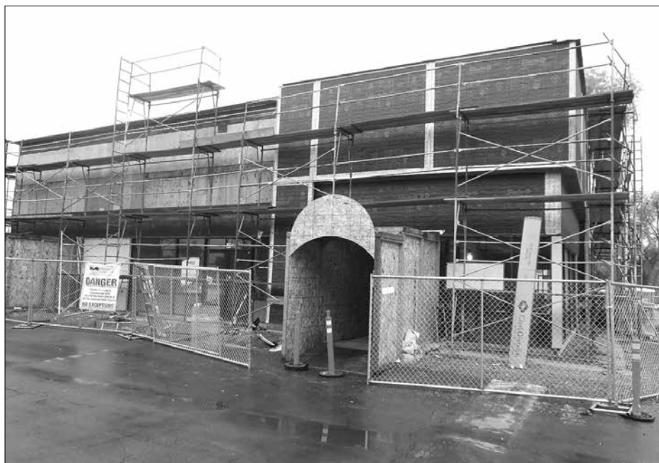
Property held by Merlone-Geier undergoing a renovation at Sunrise Village Shopping Center at 7855 Madison Avenue in Citrus Heights.
