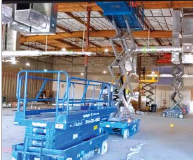
Interior work being conducted on the new plasma center at the former Dimples Records store at 7830 Macy Plaza Drive in Citrus Heights.
