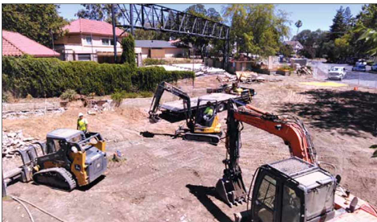
Construction crews prepare the terrain for Measure J improvements, which will include a new theater building and an enhanced Clubhouse, at Fair Oaks Village Park Plaza. Photo courtesy of FORPD/SENSERA Systems
