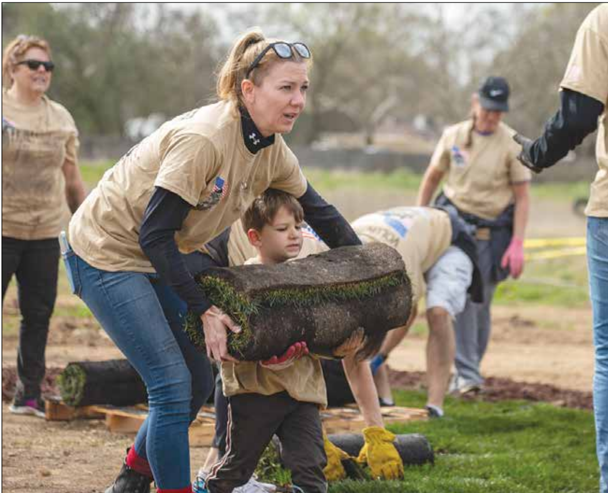
Volunteers and 'Homes for our Troops' workers spent a previous week landscaping the house as the final touches were made to the marine's new home. Photo: Cathy Kurtz photography
