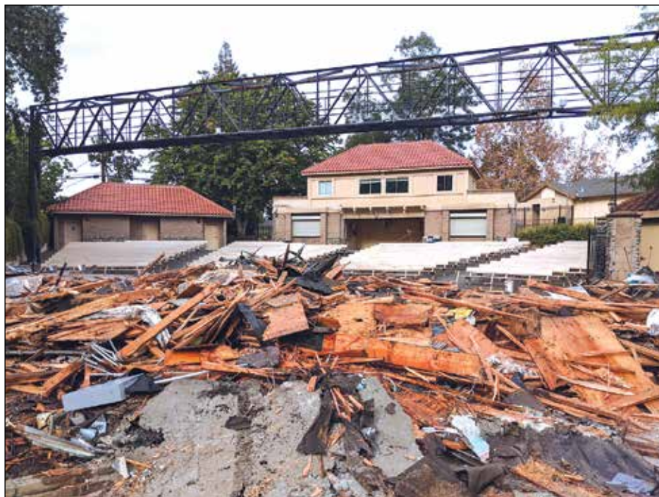
On October 7, the theatre building was demolished, making room for the planned renovation, which is funded by the Measure J bond.
