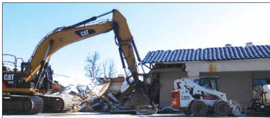
The complete clearing of the 17,200-square-foot site formerly occupied by Benihana restaurant should be done by March 31. Photo by Thomas J. Sullivan
