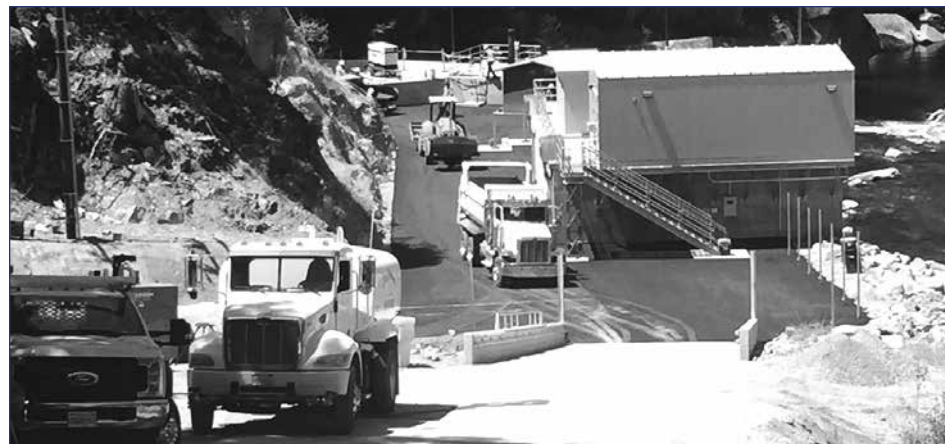
The new South Fork Powerhouse on the Upper American River is now operational and produces 2.7 megawatts of renewable power. The new hydroelectric power station includes a boating flow release facility that provides more accurate and safer recreational water flows for boaters. Photos: SMUD
