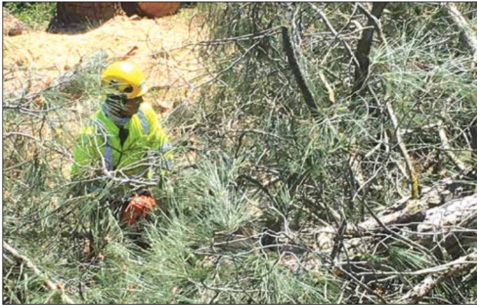
SMUD contract tree pruning workers clear high-fuel vegetation and brush under and near high-voltage transmission lines in Rescue, El Dorado County. Photo: SMUD
