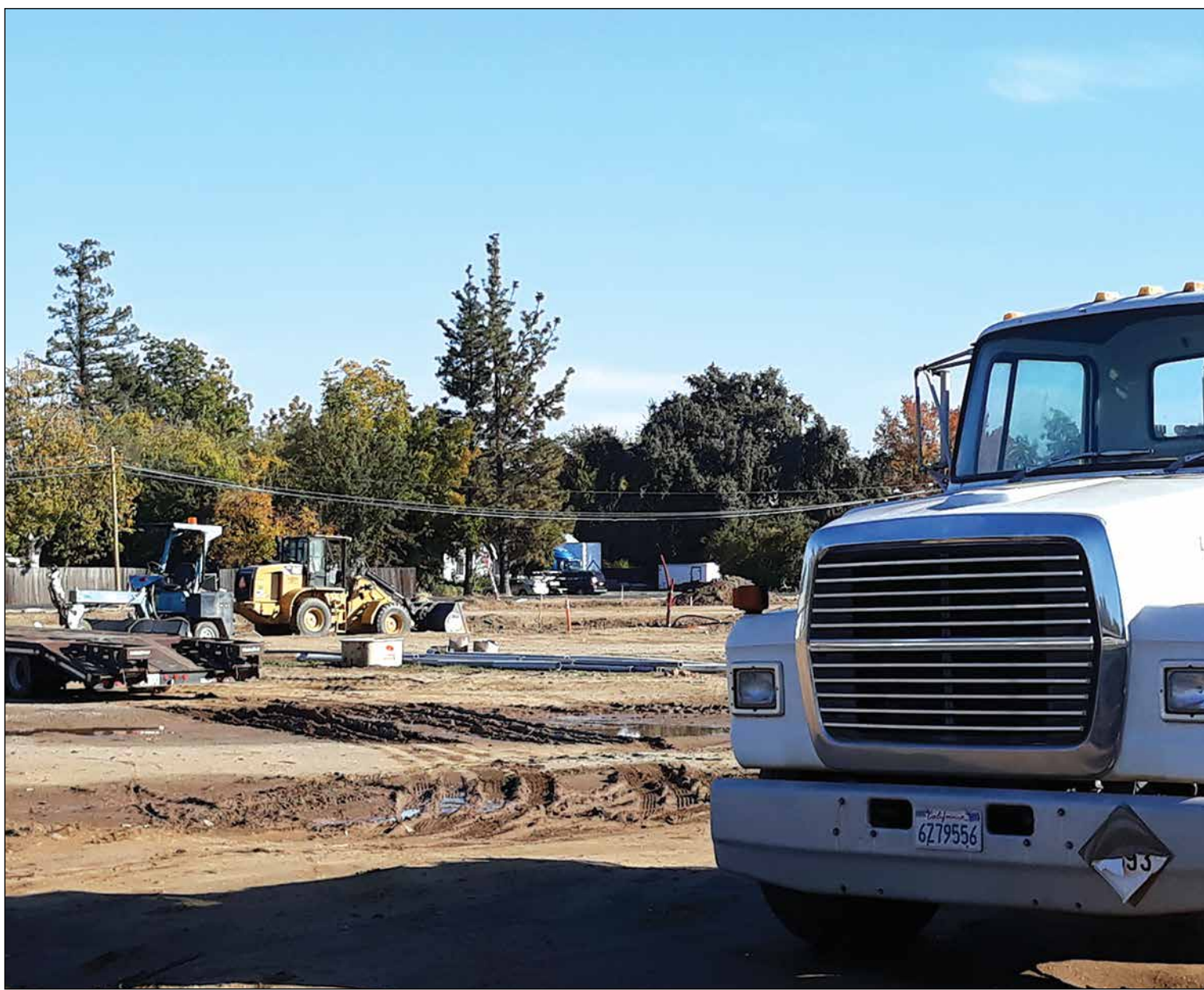
Heavy equipment has been a fixture on the Steffen Estates site for months as the infrastructure for the new housing development goes in.
