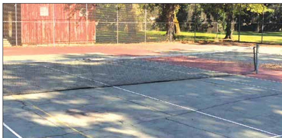
This 'before' picture of the tennis courts at Manuel Vierra Park illustrates the deteriorating condition of the courts before construction began to refurbish them. Photo courtesy of Dave Harden
