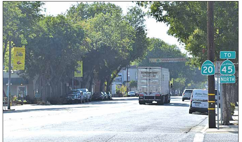
The main thoroughfare through Colusa is undergoing roadwork through the month of October. Photo courtesy of Caltrans
