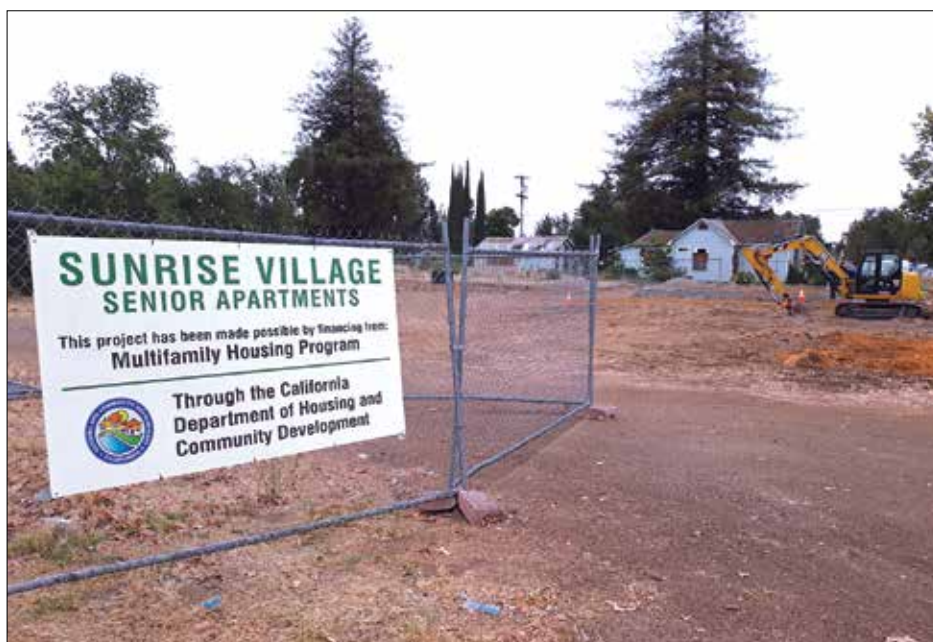
The future entrance to Sunrise Village Senior Apartments is currently the focus of the Caltrans and its SHOP project. Seen here is the current access from SR-99, where construction crews are accessing the development currently in progress.
