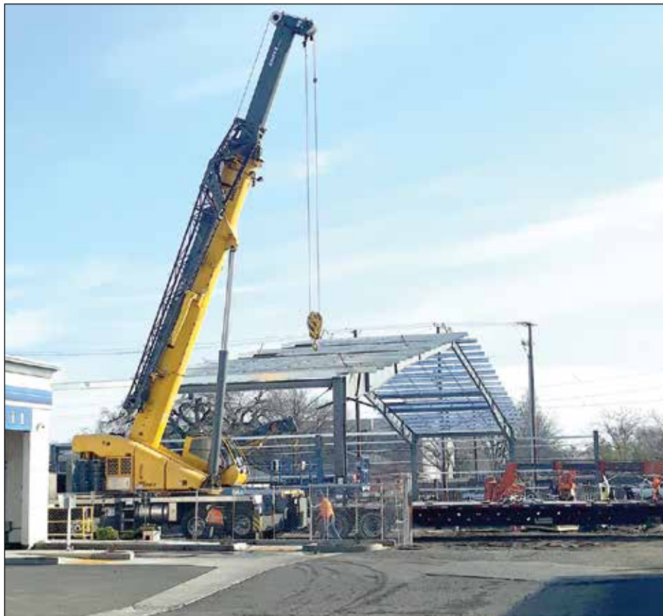
Starting to see some progress on the new Savmor store. Last week large cranes put the building's roof in place. Photo by Seti Long
