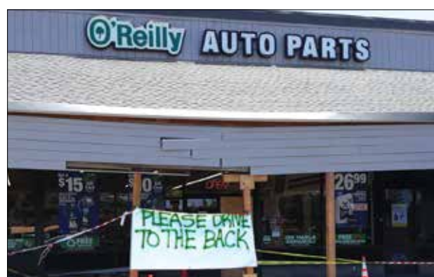
Days after the incident, damage is still visible to the O'Reilly Auto Parts store front after an SUV jumped the curb and nearly took out the store Saturday. Photo by Seti Long
