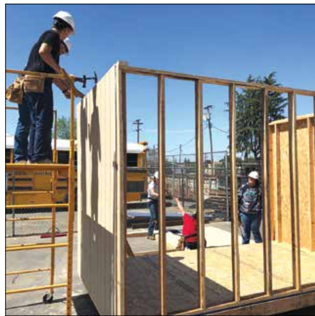
That's a nice shed!! Gridley AG students work together on the CIEF Design and Build project. Photo provided by GHS Ag Department
