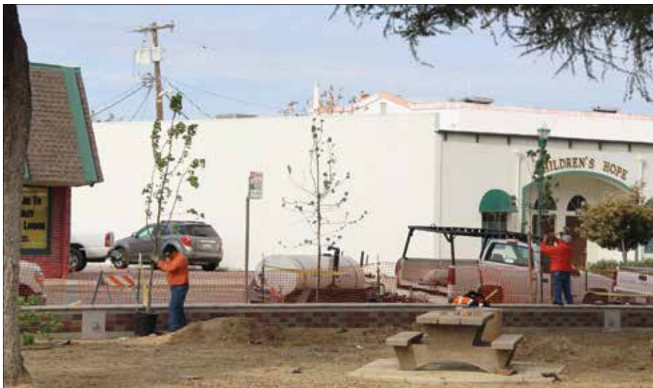
DADDOW PARK COMING TOGETHER - Thanks to the City of Gridley's Public Works, Daddow Park is nearing completion. Trees were planted this week and electrical and lighting are completed. Sod planting will be next in early April. (Photo by Lisa Van De Hey)
