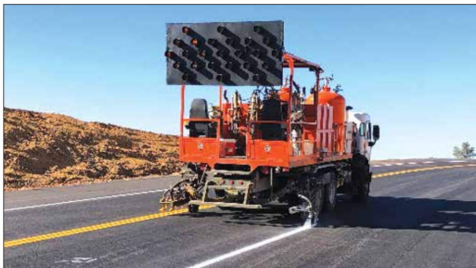
Detour is set for highway access from Steffen Trail, Valhalla Way. Photo CalTrans
