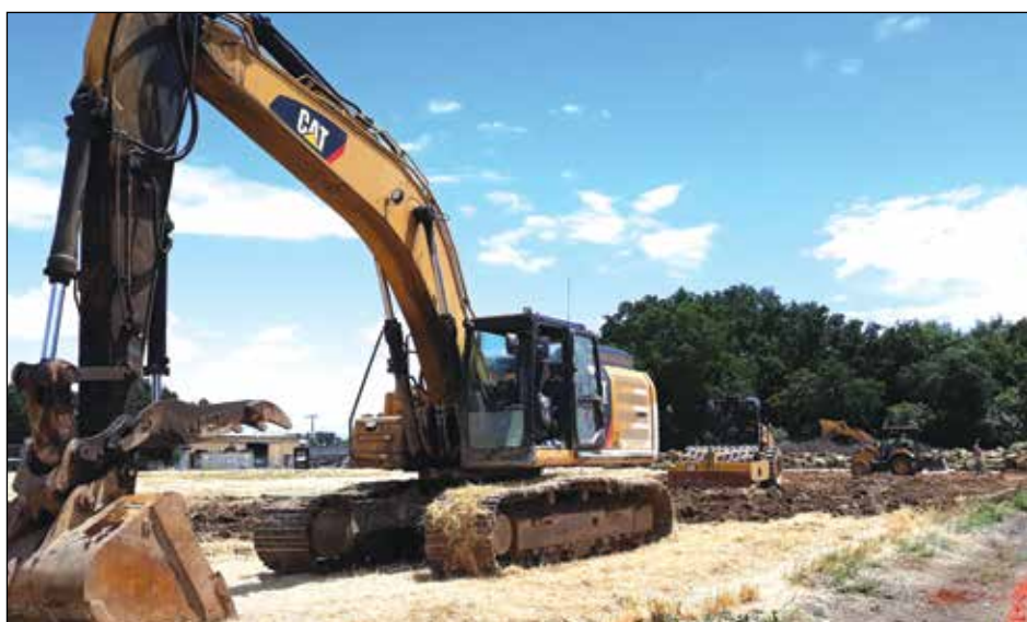
Construction of the FEMA temporary housing, which will leave the city with new permanent infrastructure, is a boon to Gridley's economy
