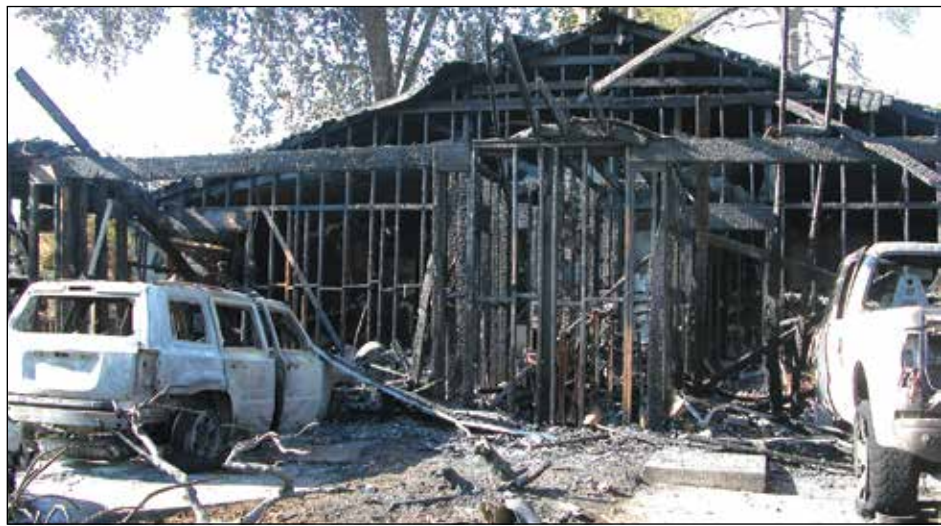
The morning hours show the damage caused by the fire at the Carmichael duplexes. Photo by Patrick Larenas
