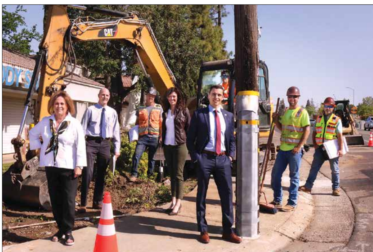
Supervisor Susan Peters (left), transport engineers Steve White and Melissa Wright, and Carmichael Chamber of Commerce President Jim Alves visit works that begin the last phase of Fair Oaks Boulevard improvements. Begun in 2013, the three-part project will be completed late 2021.
