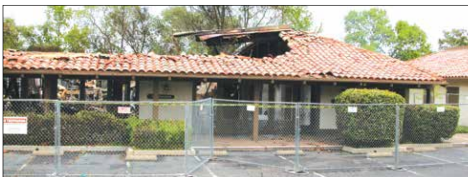
The remains of the burnt building located near the intersection of Marconi Avenue and Fair Oaks Boulevard. Photo by Patrick Larenas
