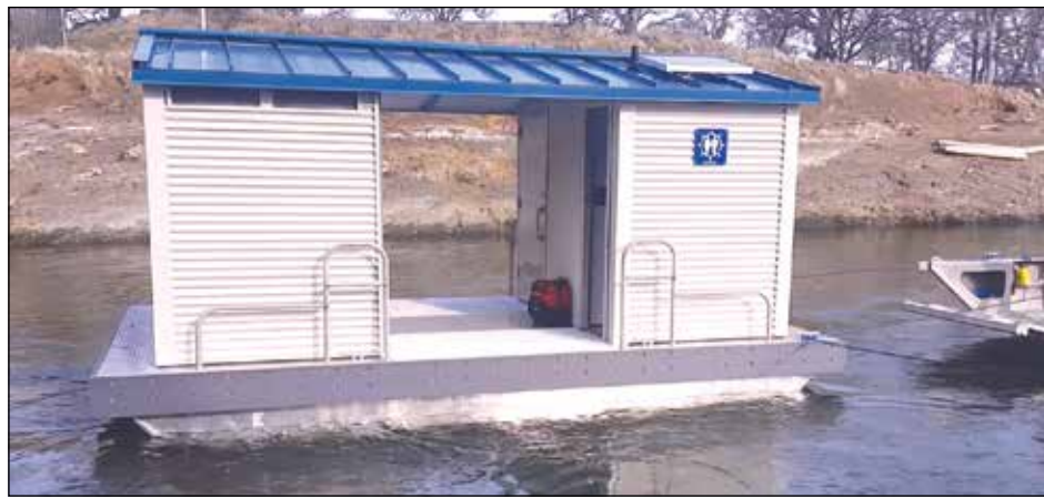
Floating restroom shown during December 2019 deployment at Lake Berryessa. Each ADA compliant unit holds about 500 gallons of sewage. Photo courtesy California State Parks
