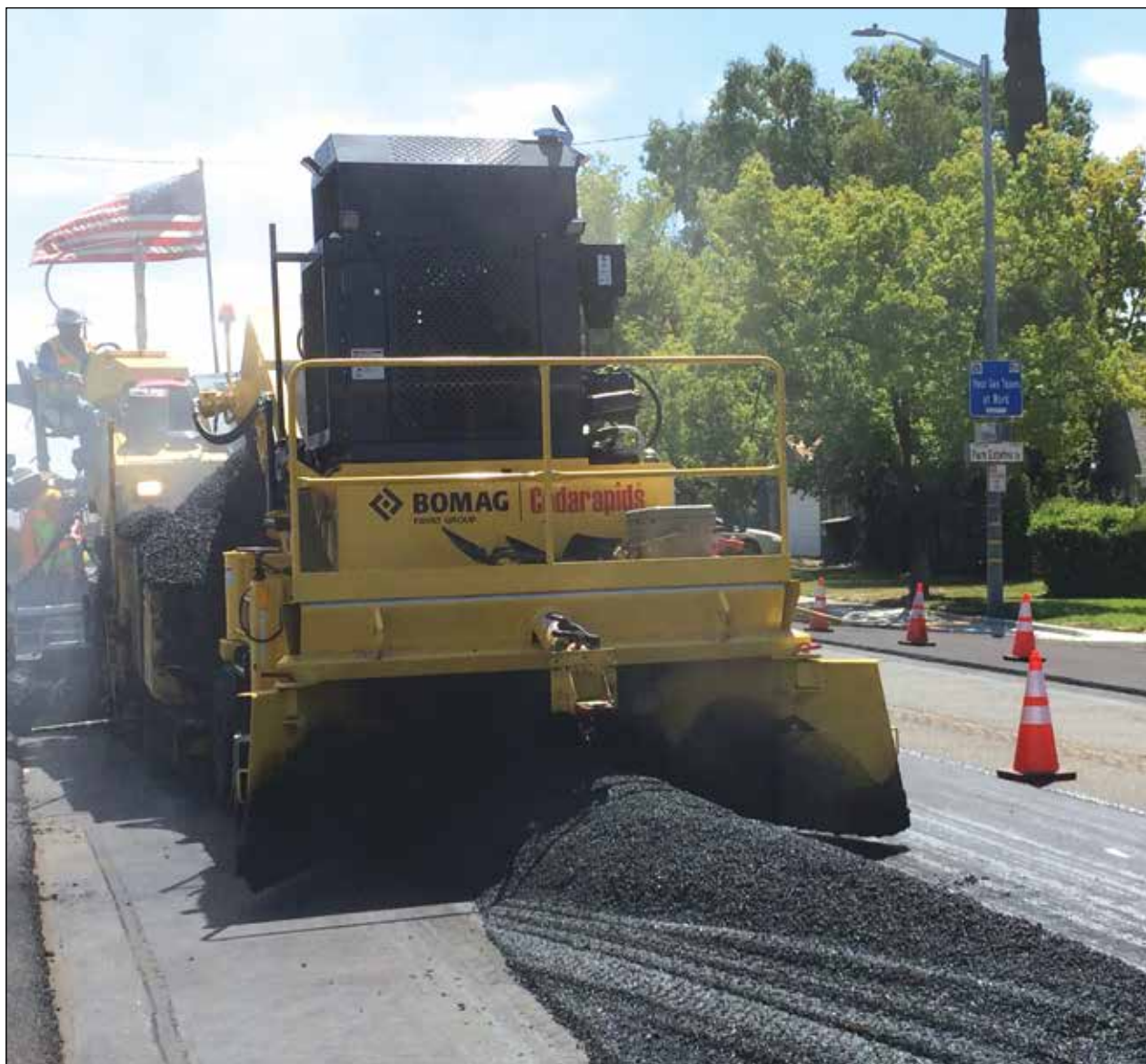
Image of a road repair crew filling in trenches on one of our roadways. Photo courtesy of Sacramento County.
