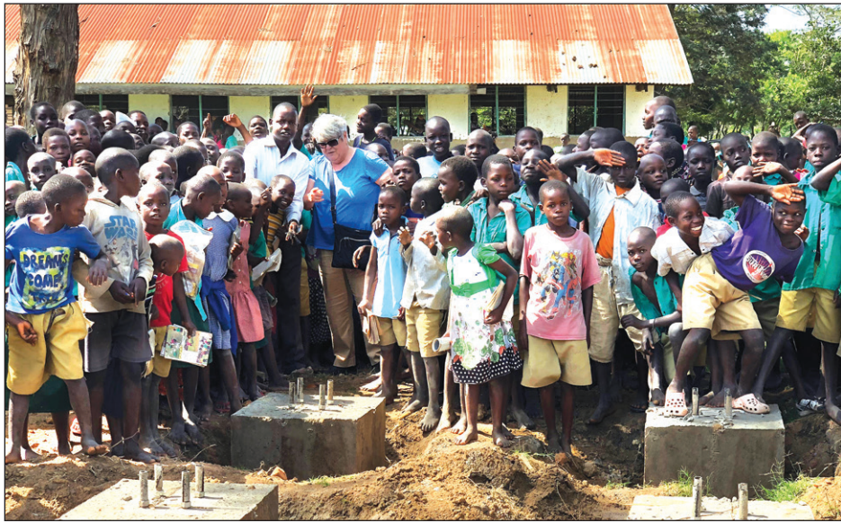
Richard Olebe's wife Margaret joined Ugandan children as they watched water tank construction at their school. Photo courtesy Richard Olebe.
