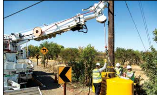
SMUD has seen an increase in “car-pole” accidents in recent years, so the electric utility is installing some measures to mitigate damage to power poles and other electrical equipment. The work is part of SMUD’s efforts to enhance public and worker safety and the SMUD grid’s reliability. Photo courtesy SMUD
